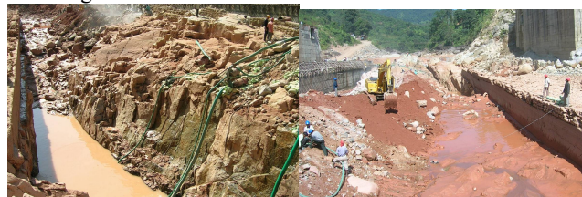
Fig. 4 Shear seam at MyntduLeshka hydro-electric project, Meghalaya
