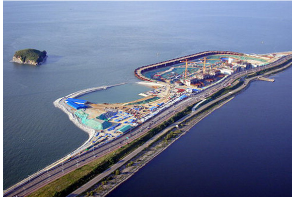
Figure 3 - South Korea's 254MW Sihwa Lake Tidal Power Station [Source: Power Technology]
